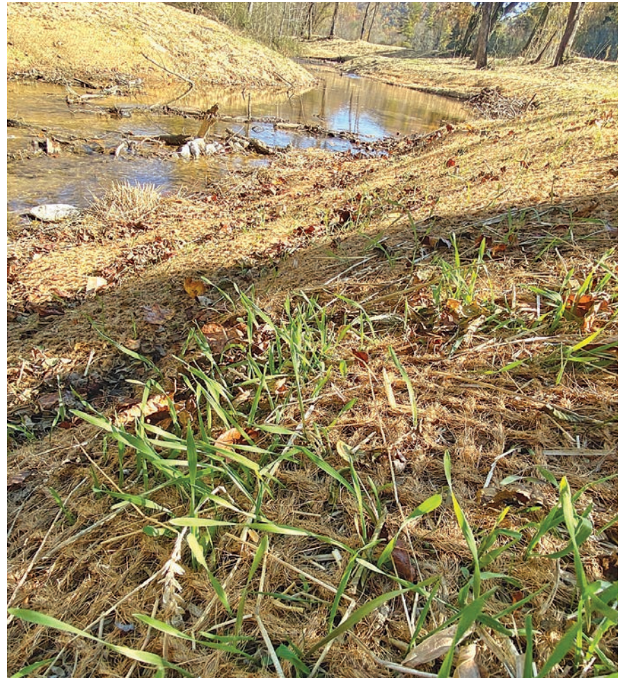
Grasses sprouting through the bank stabilization fabric are just the first of more vegetation plantings yet to come, including a variety of native trees and shrubs.
